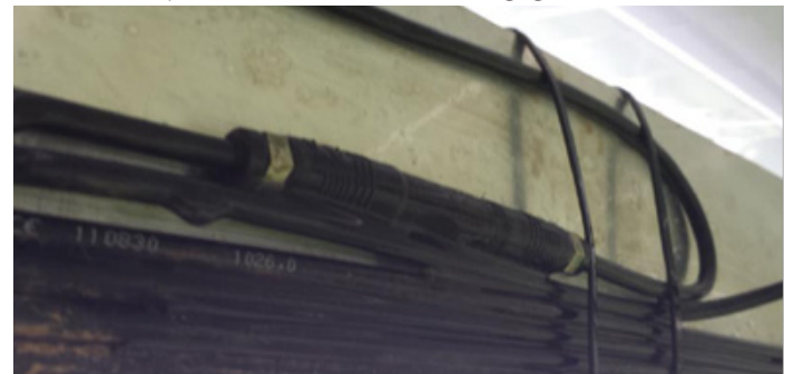
Fig. 10: Fastening of the connector tight to the mounting structure can cause moisture build up between connector and rail, damaging the connection
