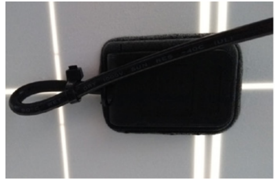
Fig. 9: Example of cable exiting the junction box at an extreme angle
