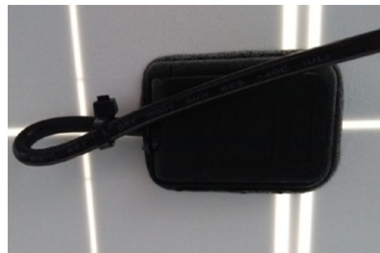
Fig. 10: Example of cable exiting the junction box at an extreme angle
