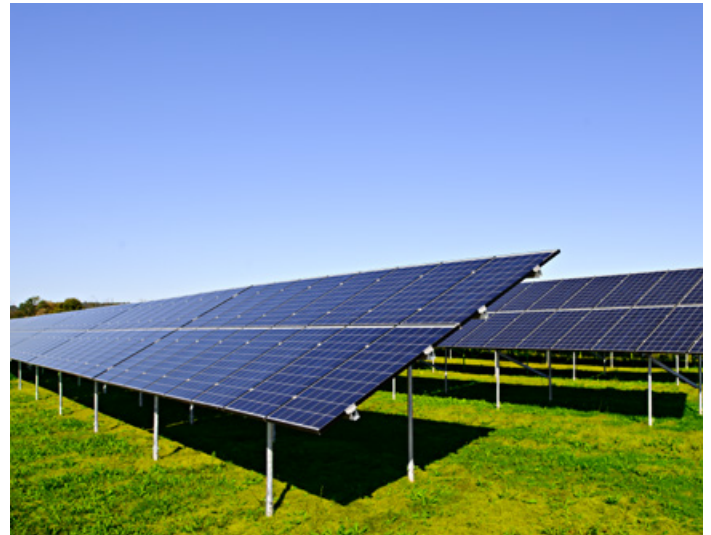
Fig. 3: A clean and functioning solar installation
