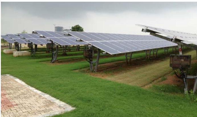
The complete system installed at PDDU campus
