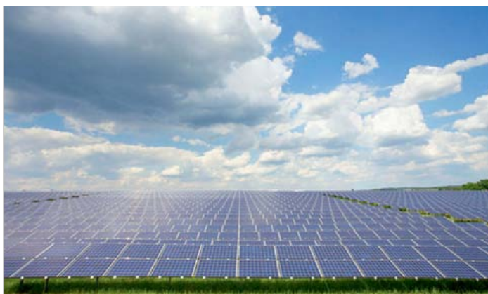
The 5.72 MW solar park with REC panels installed in Richelbach, Germany
